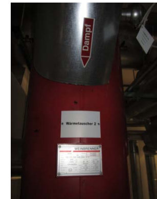
Addition heat exchanger
